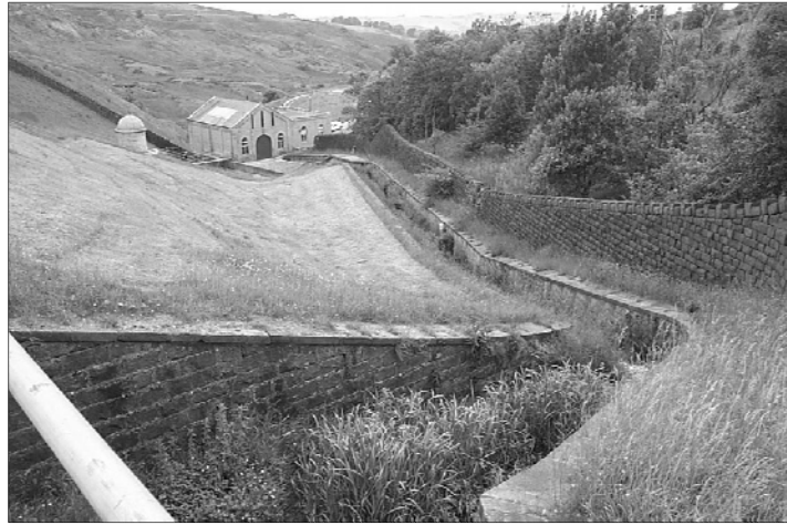
Figure 3. View from the overflow weir showing the existing spillway falling down the embankment to the pump house.
